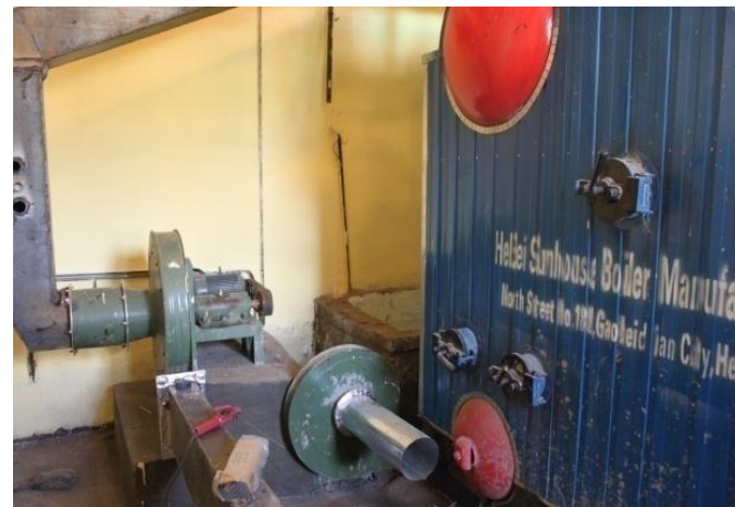
Central heating system
