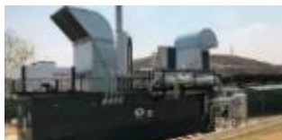
Power Generation with Methane Gas Recovery System, NTTDATA, Mexico
