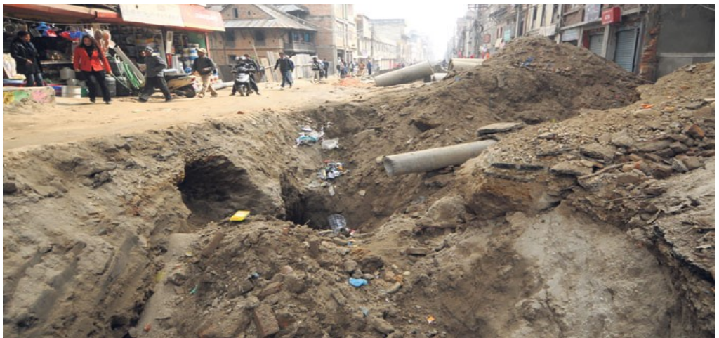
The Maitidevi-Dillibazar road section currently under construction pictured on Sunday. (Dipesh Shrestha/Republica)
